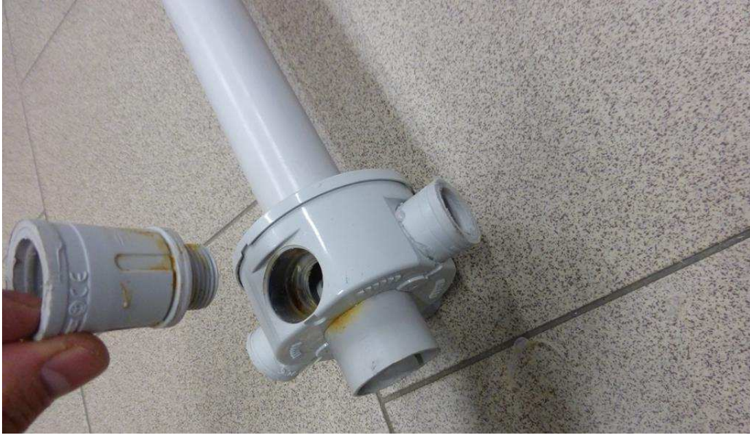
Fig. 5. Installation of the round junction box on the conduit (bottom part of the drifter).
